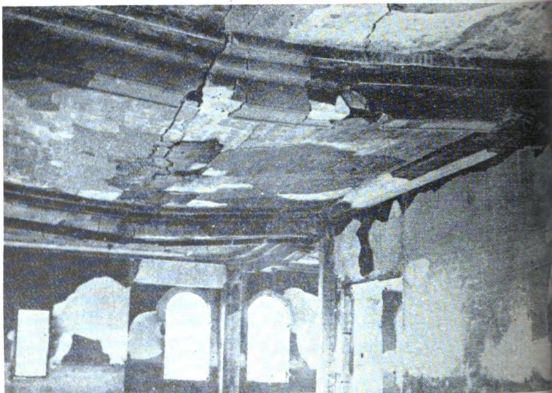
Figure 5.54a. Upper photo: Reinforced-concrete frame building, 700 feet from ground zero, 2,100 feet from point of explosion; external walls intact. Lower photo: Interior of above burned out; note sagging of roof and spalling of plaster by fire.
